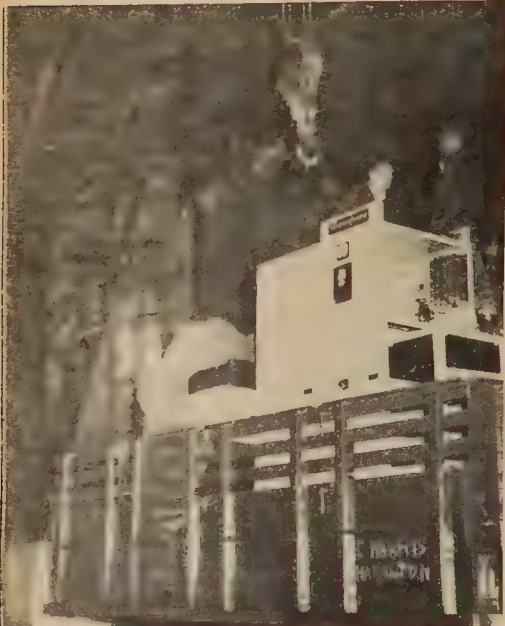
Here the new 60-cycle switchboard for Hart House is seen being unloaded by a huge crane at the side door of Hart House late last night. The electric switchboard, weighing 7,000 lbs., is for the 400 volt power sub-station being installed in Hart House for the changeover from 25 to 60 cycle.
